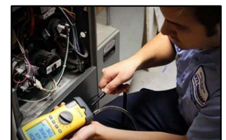
Industrial & Residential / Facility Services
